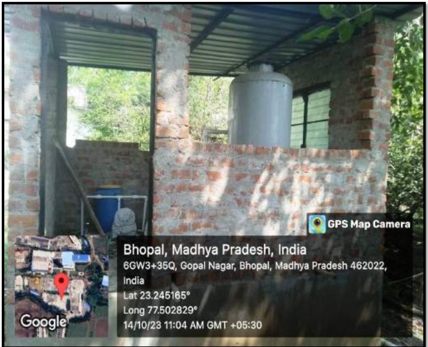
GPS PHOTO OF STP PLANT
